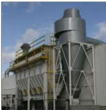
Bag filter, cyclones
